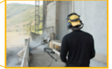
Robot operating on the platform removing concrete from a bridge substructure. L'Aquila, Italy.
